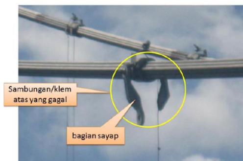
Figure 1. Broken clamp connection
