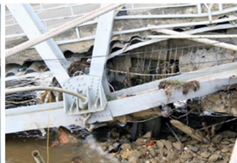
Figure 2. Lower clamp collapse
